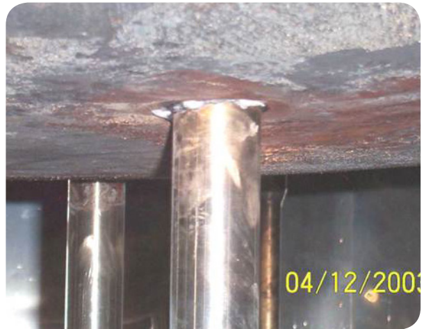
Bare-Metal Visual image of boron deposits from confirmed leaking BMI.
